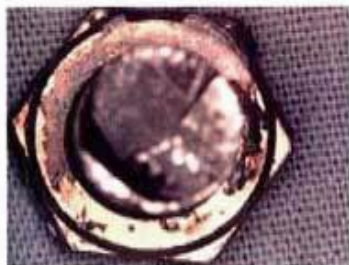
(Photo: H F Consultants) FIGURE 1b. Underside of fractured bolt head showing lack of damage to plating. Thrust face of associated nut showed similar lack of damage
